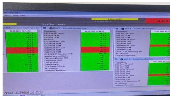
Gambar 12. Pengecekan meter reading peralatan
